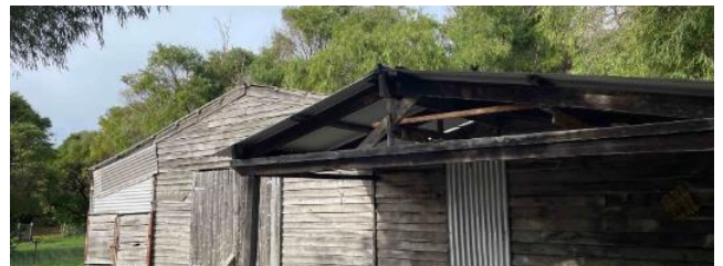
Figure 13: Salmon fishing net shed (circa 1947), being the oldest structure on the reserve
