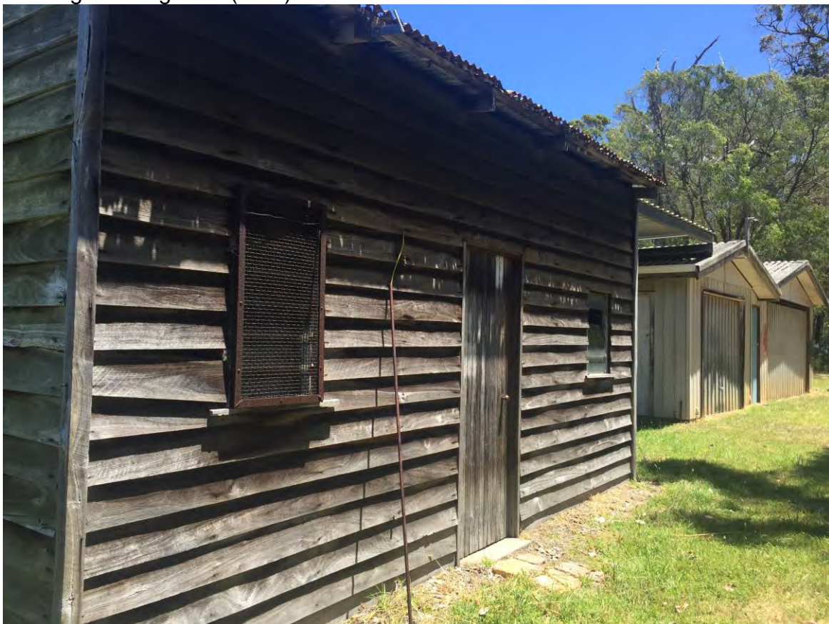
Northern elevation of wooden outbuilding to be retained. Outbuilding in the distance (west) to be removed.
