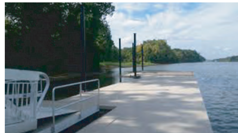
IMAGE: FLOATING JETTY
