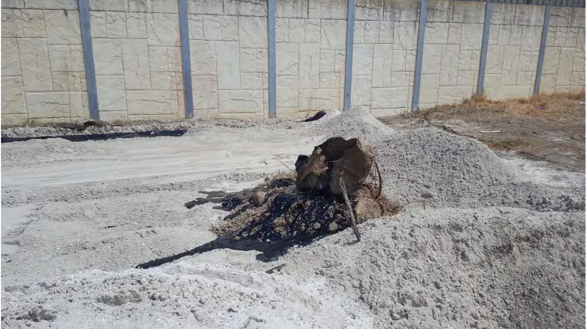
Bitumen Drum in plastic lined containment area
