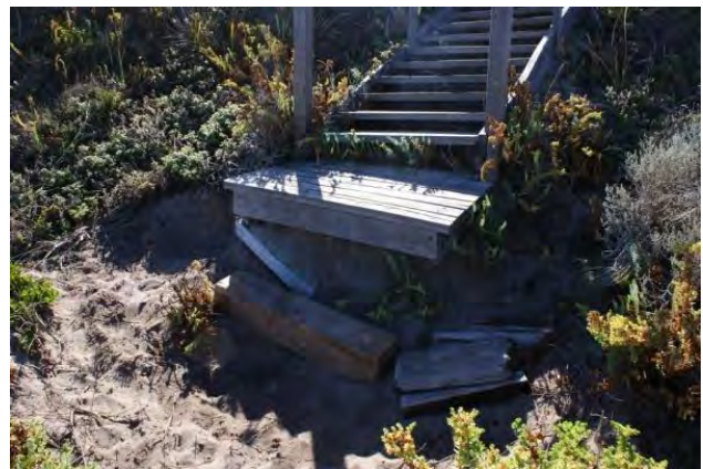
Picture of the broken timber step at Back Beach
