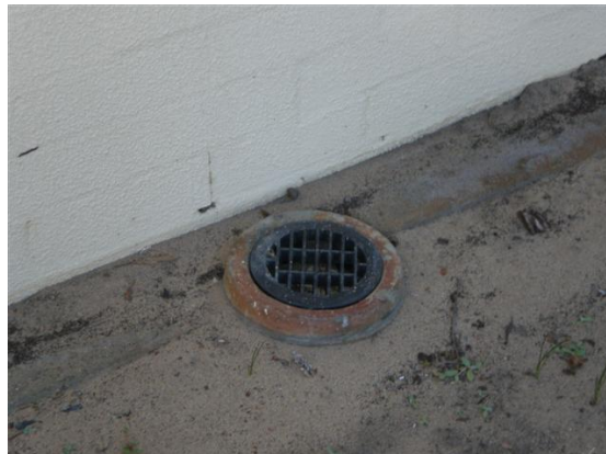
Overflow Relief Gully
