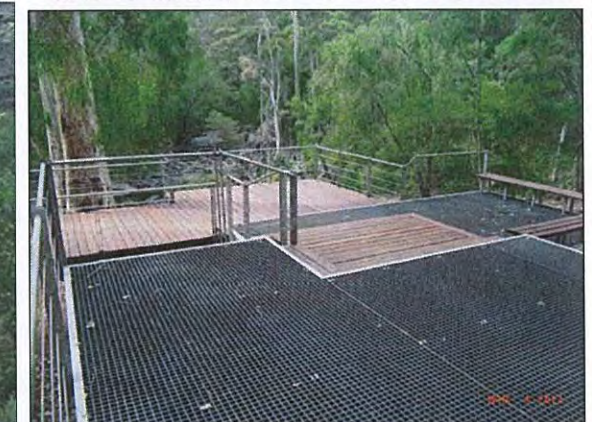
MIX OF MATERIALS - HANDRAILS
